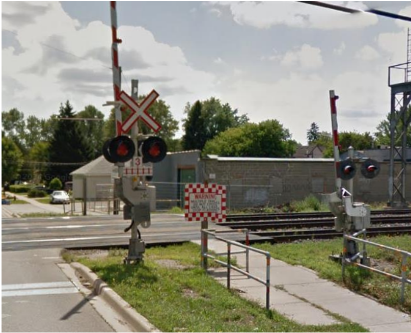
Flashing lights and a gate
