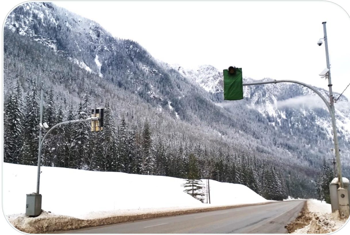
Variable Speed Limit System
